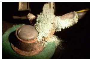
Corroded battery terminal
